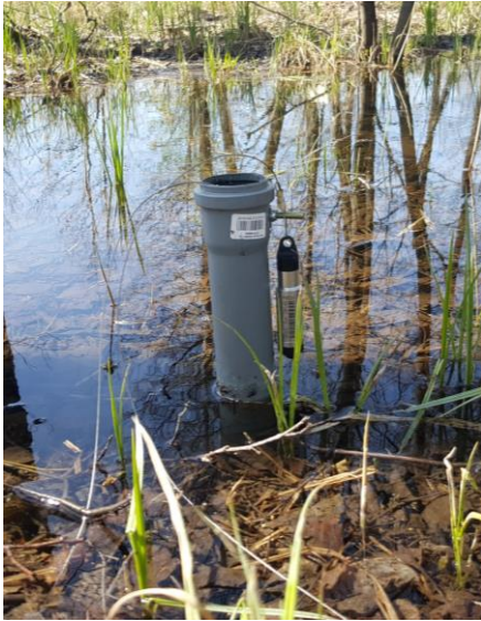
A system of hydrological monitoring was installed.
